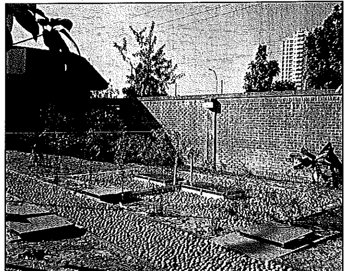
Cromaglass Model CA-60 treating 6,000gpd of wastewater from the embassy compound - Installed December 1999.
