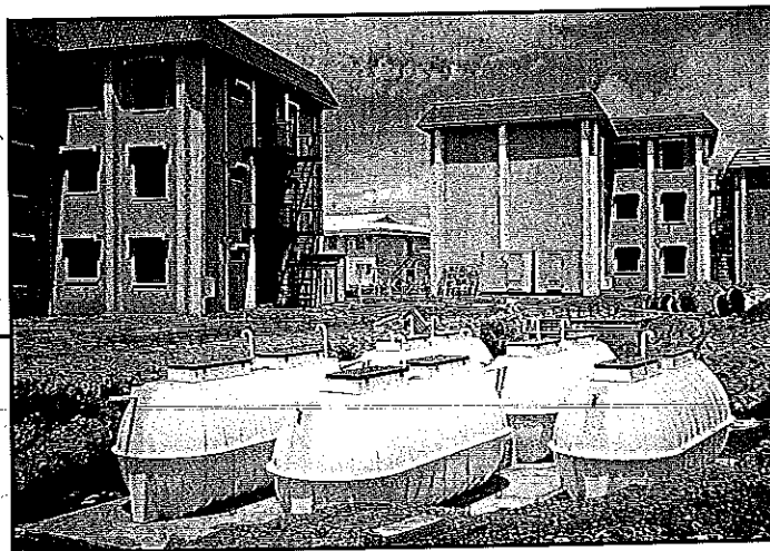
Pagbilao Treatment System located at Staff housing Quarters – Powerplant nearby. Two Model CA-150 Modules and 5,000 gallon sludge processing system.
